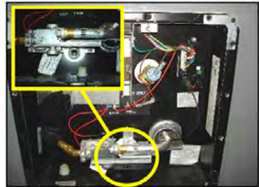
Fig 1: Water heater drain plug
